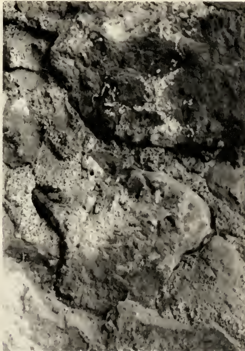
Fig. 29. Efflorescence on sandstone 1.5' (46 cm.) above grade at northeast wall of apse.
